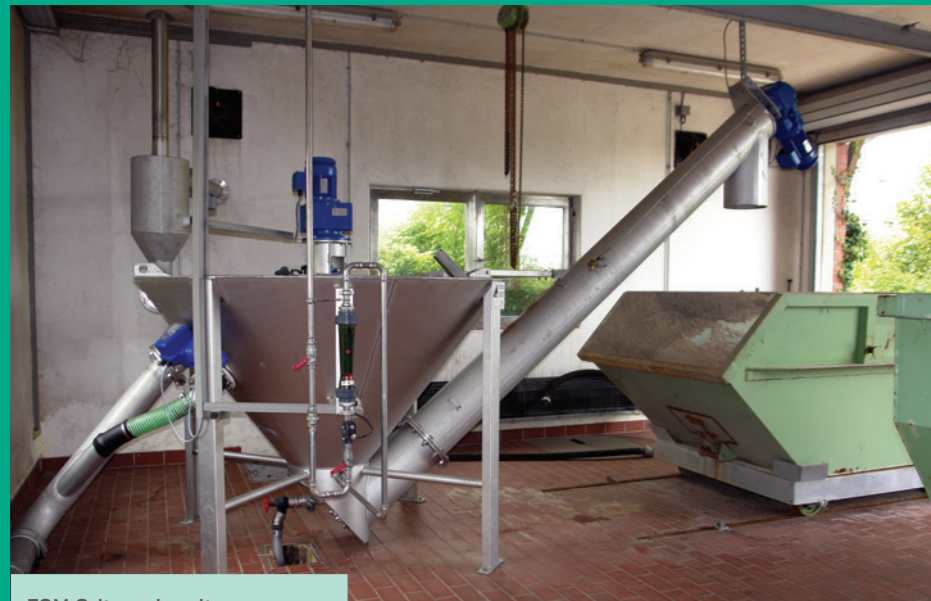
FSM Grit wash unit
