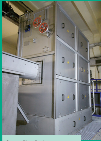
Center Flow Rechen
